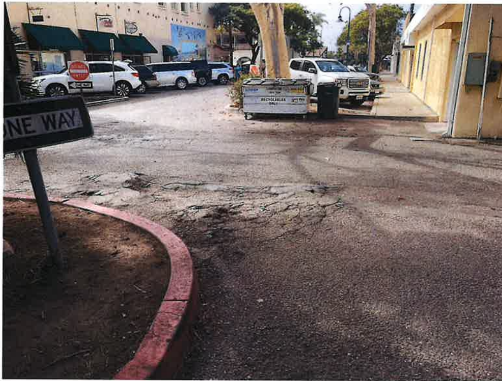
Figure 25: Lot 2 Pavement Conditions
