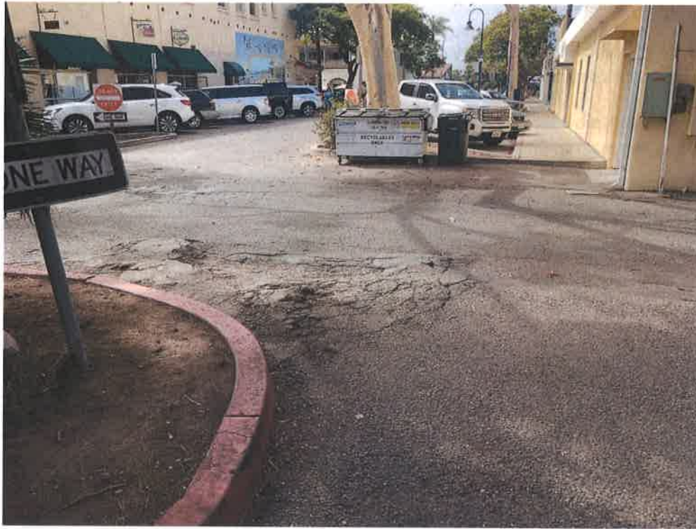
Figure 25: Lot 2 Pavement Conditions
