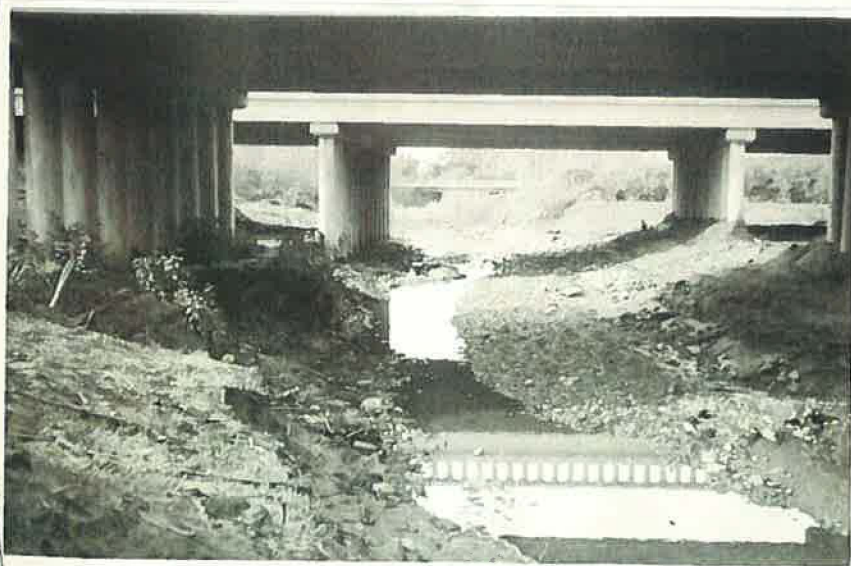
BRS 143-8 Same, DS under bridge showing misalignment of piling with channel of retreat
