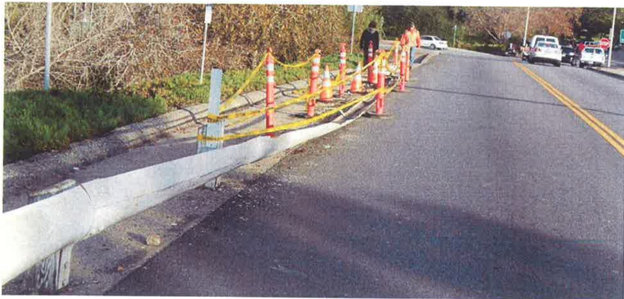
Figure 2. Santa Ynez Guardrail Damage
