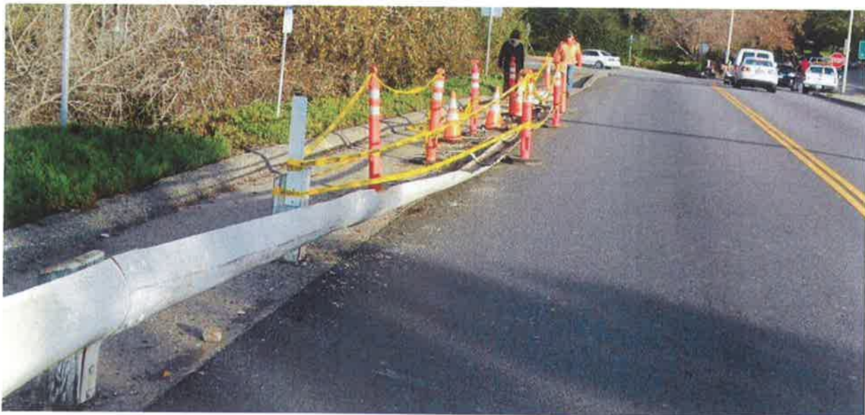
Figure 2. Santa Ynez Guardrail Damage
