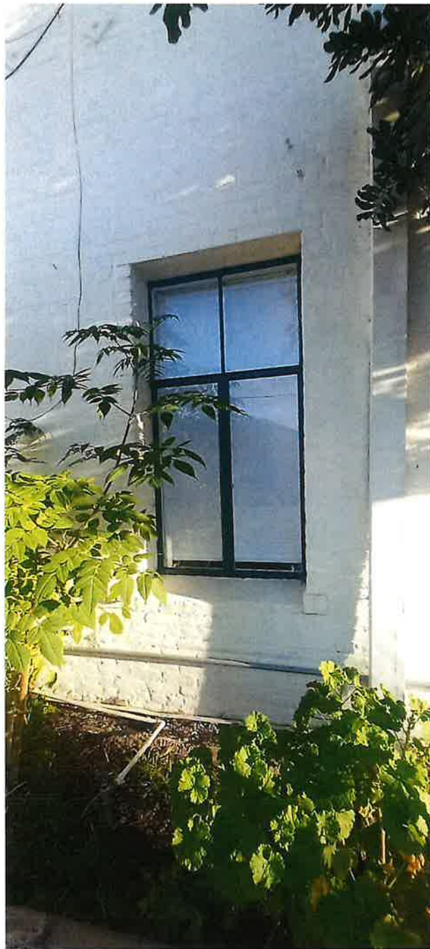
Exhibit 24, Non-contributing metal frame window at the south end of the west elevation (November 2023)
