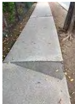
Hazard 26: 1275 Casitas Pass Rd
