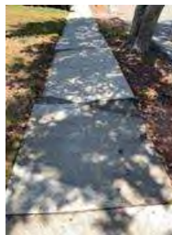
Hazard 17: 5439 Dariesa St
