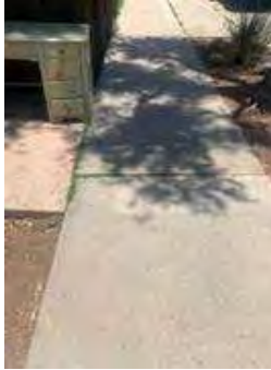
Hazard 1: 1476 Haida St
