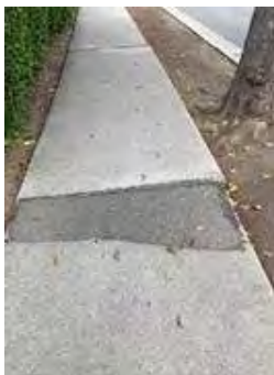
Hazard 25: 1335 Casitas Pass Rd
