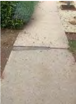
Hazard 6: 1509 Jay St
