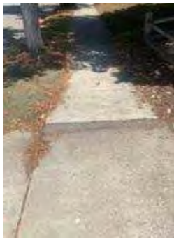
Hazard 13: 5423 Shemara St
