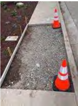
Hazard 22: 5201 Ogan Rd
