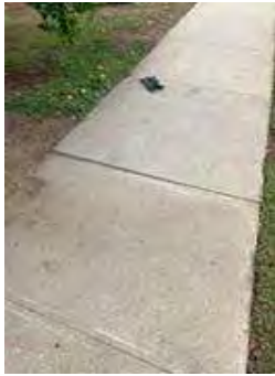
Hazard 13: 1453 Casitas Pass Rd
