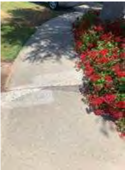
Hazard 5: 1483 Alva St
