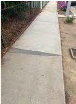
Hazard 7: 1519 Casitas Pass Rd
