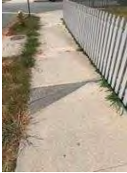
Hazard 10: 5408 Shemara St
