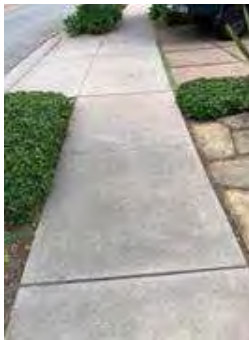
Hazard 27: 5317 Ogan Rd
