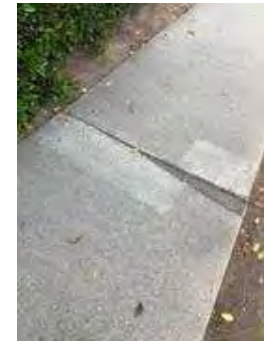
Hazard 24: 1335 Casitas Pass Rd X cut
