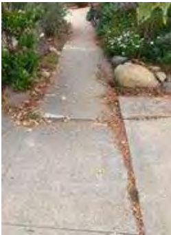
Hazard 4: 5464 Cameo Rd
