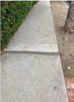
Hazard 29: 1273 Casitas Pass Rd
