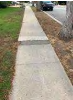
Hazard 2: 5488 Cameo Rd
