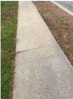
Hazard 1: 5488 Cameo Rd
