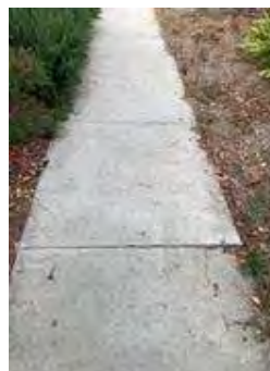
Hazard 17: 1306 La Manida St
