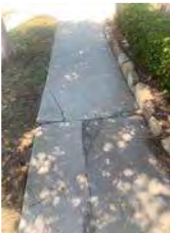
Hazard 6: 5458 Dariesa St
