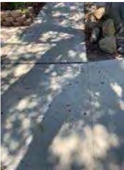
Hazard 8: 5410 Dariesa St
