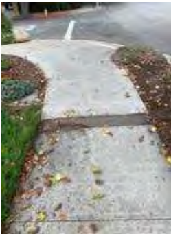
Hazard 5: 1529 Casitas Pass Rd
