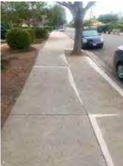
Hazard 8: 1493 Andrea St
