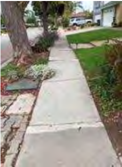
Hazard 11: 5421 Cameo Rd
