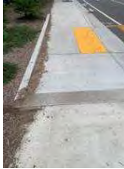
Hazard 2: 5002 Pacific Village Dr
