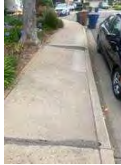
Hazard 11: 5482 Granada Way
