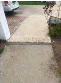
Hazard 2: 1470 Andrea St
