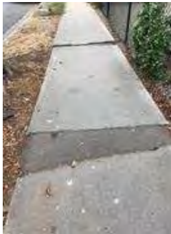
Hazard 22: 1505 Casitas Pass Rd
