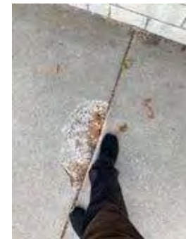
Hazard 18: 5382 Santa Rosa Ln
