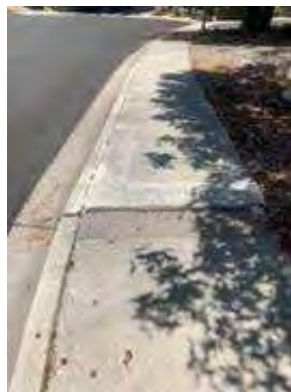
Hazard 1: 5378 Santa Rosa Ln
