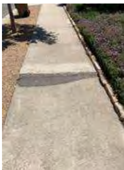
Hazard 16: 5423 Dariesa St
