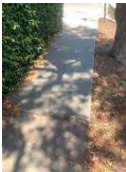
Hazard 7: 1477 Noma St
