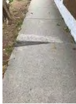
Hazard 20: 5383 Ogan Rd
