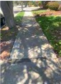
Hazard 5: 5444 Dariesa St
