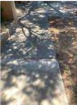
Hazard 2: 1539 Casitas Pass Rd
