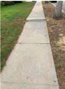
Hazard 3: 5476 Cameo Rd X cut
