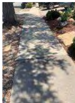
Hazard 17: 5451 Shemara St
