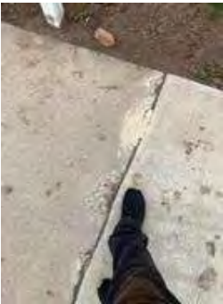
Hazard 6: 1529 Casitas Pass Rd
