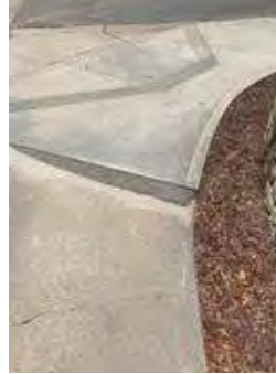
Hazard 2: 1476 Haida St
