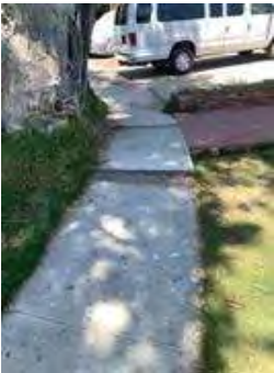
Hazard 3: 1554 Lisa St
