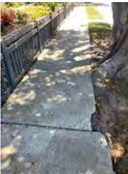
Hazard 9: 5410 Dariesa St
