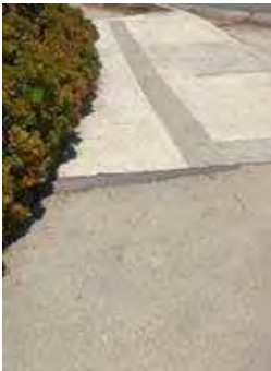
Hazard 1: 1478 Alva St
