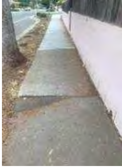
Hazard 10: 1491 Namouna St
