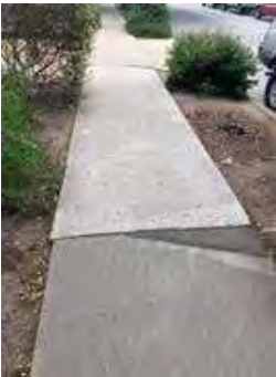
Hazard 21: 5290 Ogan Rd
