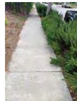
Hazard 18: 1306 La Manida St
