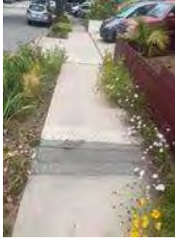
Hazard 1: 5384 Ogan Rd
