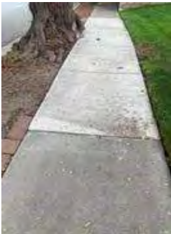
Hazard 1: 1547 Casitas Pass Rd
