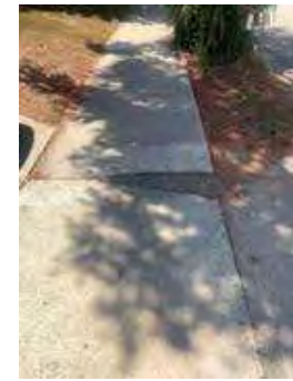
Hazard 15: 5431 Shemara St
