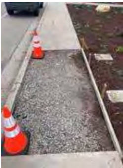
Hazard 22: 5201 Ogan Rd
