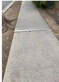
Hazard 23: 1335 Casitas Pass Rd
