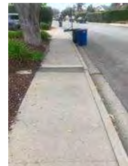
Hazard 9: 5481 Granada Way
