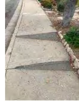
Hazard 12: 5474 Granada Way
