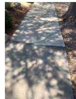
Hazard 18: 5451 Shemara StX cut
