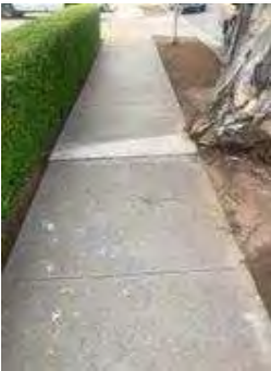
Hazard 5: 1492 Trenora St
