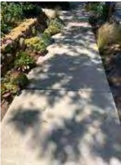
Hazard 20: 5479 Dariesa St
