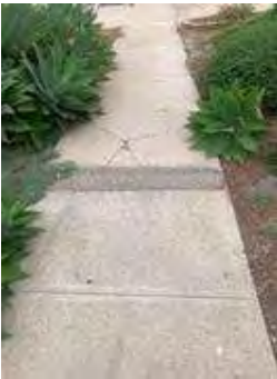
Hazard 5: 1539 Jay St
