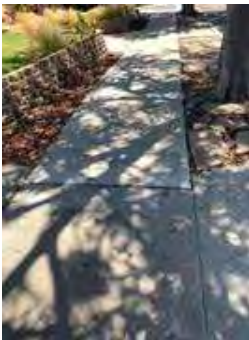
Hazard 7: 5422 Dariesa St
