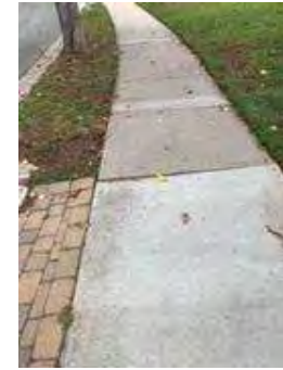
Hazard 33: 1514 Jay St
