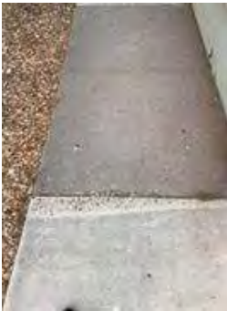
Hazard 20: 5290 Ogan Rd
