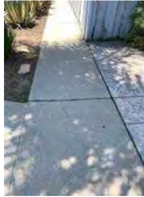
Hazard 1: 1549 Kathy St
