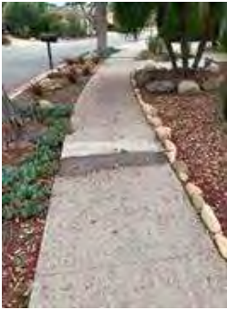
Hazard 13: 5441 Cameo Rd
