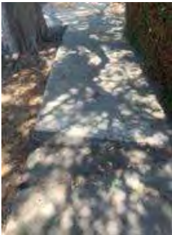
Hazard 1: 1539 Casitas Pass Rd
