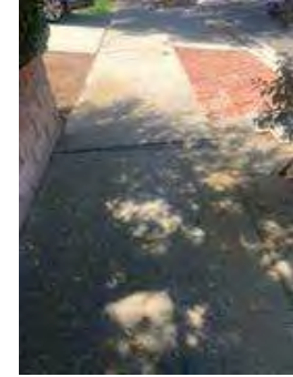
Hazard 12: 5405 Shemara St
