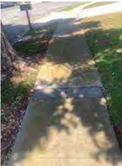
Hazard 2: 5444 Dariesa St
