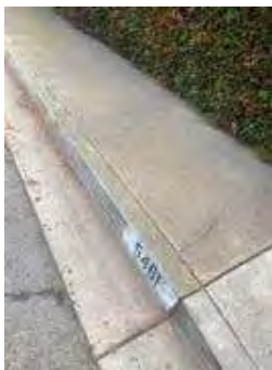
Hazard 7: 5461 Granada Way Sw^c
