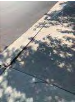
Hazard 3: 5378 Santa Rosa Ln
