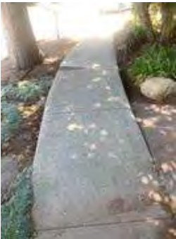
Hazard 3: 1547 Myra St
