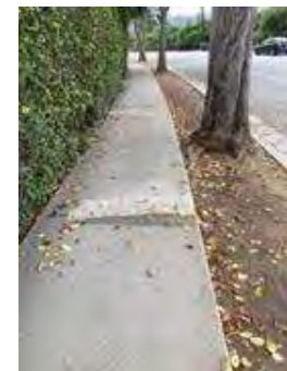
Hazard 27: 1275 Casitas Pass Rd
