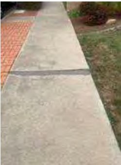
Hazard 2: 1552 Jay St
