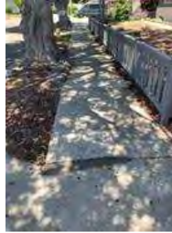
Hazard 11: 5378 Dariesa St
