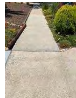
Hazard 18: 5447 Dariesa St
