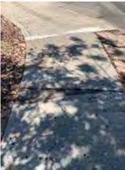
Hazard 6: 5422 Dariesa St
