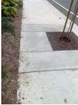
Hazard 1: 5002 Pacific Village Dr
