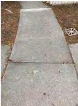
Hazard 7: 5414 Cameo Rd X cut
