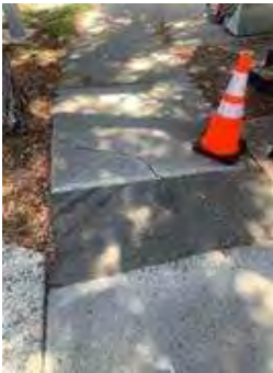
Hazard 1: 1476 Haida St
