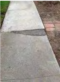
Hazard 2: 1547 Casitas Pass Rd
