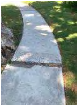
Hazard 4: 1555 Lisa St
