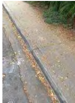
Hazard 5: 5428 Granada Way Sw^c
