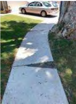
Hazard 4: 1555 Lisa St
