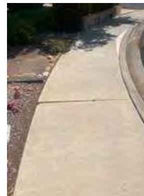
Hazard 2: 1360 LA Mesa Plz
