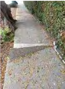
Hazard 3: 1547 Casitas Pass Rd
