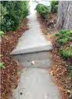
Hazard 30: 5487 Cameo Rd
