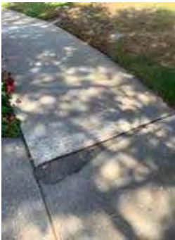
Hazard 4: 1488 Alva St
