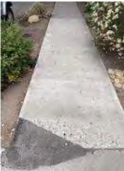
Hazard 21: 5290 Ogan Rd
