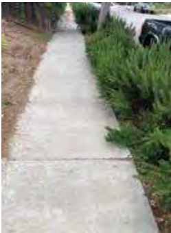
Hazard 18: 1306 La Manida St
