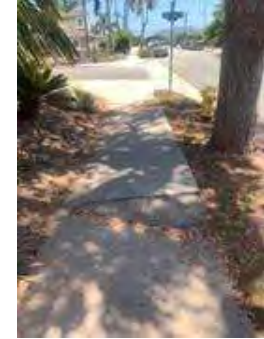
Hazard 3: 1477 Haida St
