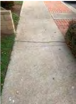
Hazard 3: 1558 Jay St
