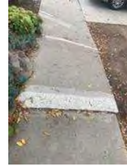
Hazard 3: 5380 Ogan Rd
