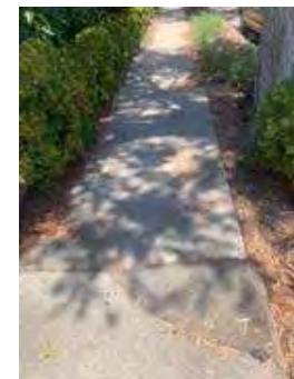
Hazard 9: 1478 Alva St
