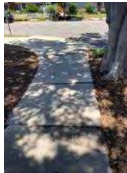
Hazard 14: 1524 Jay St
