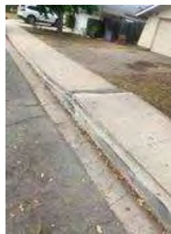
Hazard 17: 5428 Granada Way
