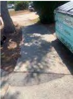
Hazard 6: 1483 Alva St
