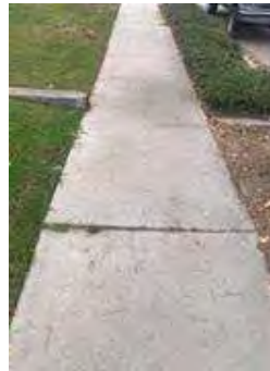
Hazard 5: 5372 Ogan Rd
