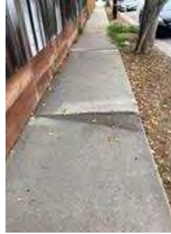
Hazard 11: 5494 Shemara St
