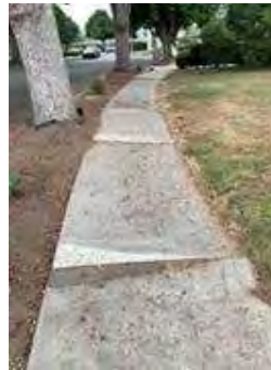
Hazard 23: 5470 El Carro Ln
