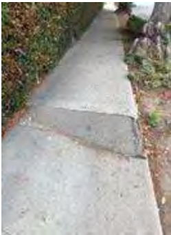
Hazard 4: 1539 Casitas Pass Rd
