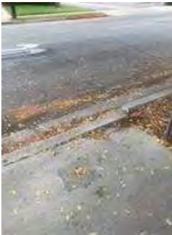
Hazard 1: 1500 Linden Ave C^sw
