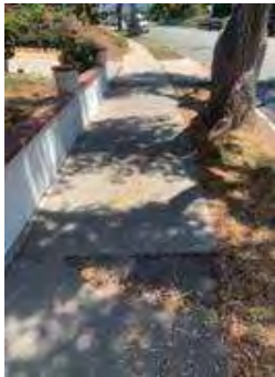
Hazard 4: 1478 Noma St
