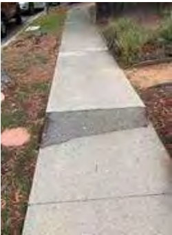
Hazard 6: 5420 Cameo Rd
