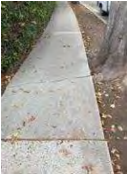
Hazard 28: 1275 Casitas Pass Rd
