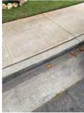
Hazard 1: 5415 Hales Ln Sw^c
