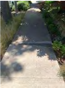
Hazard 21: 5479 Dariesa St
