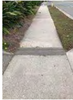
Hazard 14: 1453 Casitas Pass Rd
