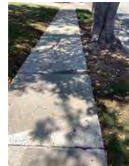
Hazard 15: 5417 Dariesa St
