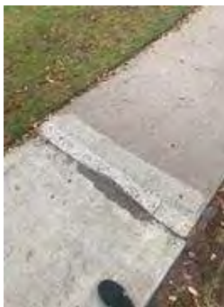
Hazard 7: 5368 Ogan Rd
