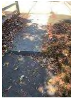
Hazard 14: 5423 Shemara St
