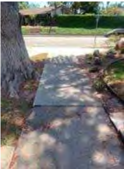
Hazard 3: 1477 Haida St
