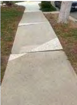
Hazard 3: 1491 Namouna St
