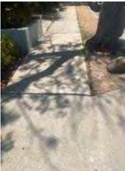
Hazard 3: 5476 Dariesa St
