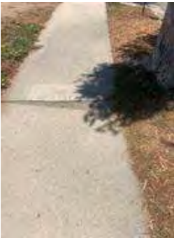
Hazard 20: 5459 Shemara St
