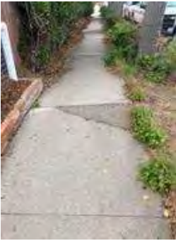
Hazard 32: 5487 Cameo Rd
