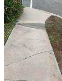
Hazard 12: 1453 Casitas Pass Rd
