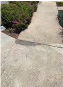
Hazard 19: 5463 Dariesa St
