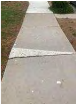
Hazard 2: 1491 Namouna St
