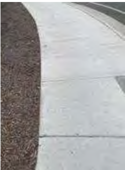
Hazard 23: 5001 Pacific Village Dr
