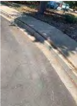
Hazard 2: 5378 Santa Rosa Ln
