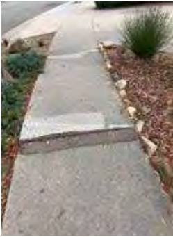
Hazard 14: 5441 Cameo Rd
