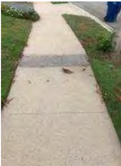
Hazard 1: 1514 Jay St
