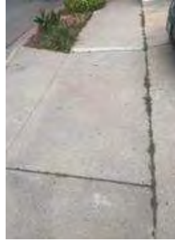
Hazard 2: 5384 Ogan Rd
