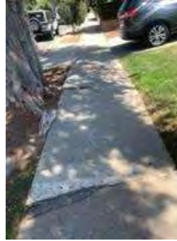
Hazard 11: 5405 Shemara St
