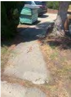
Hazard 6: 1483 Alva St
