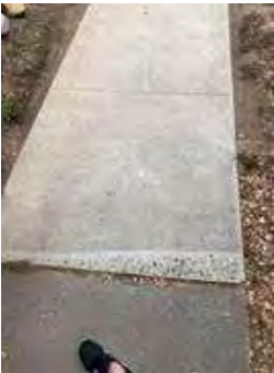
Hazard 20: 5290 Ogan Rd
