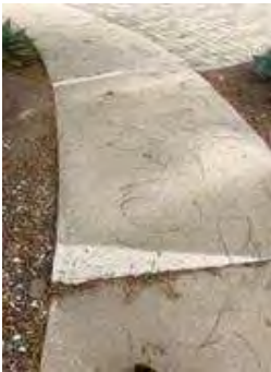
Hazard 5: 1472 Namouna St
