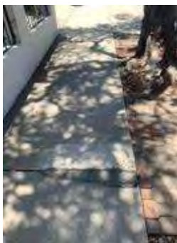
Hazard 16: 5445 Shemara St
