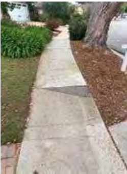
Hazard 5: 5444 Cameo Rd
