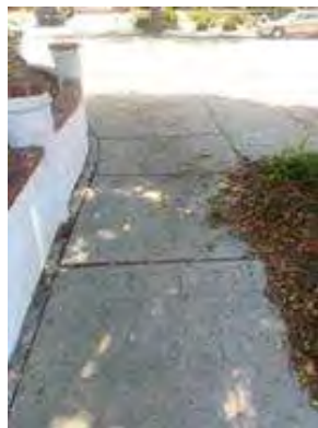
Hazard 1: 1478 Noma St
