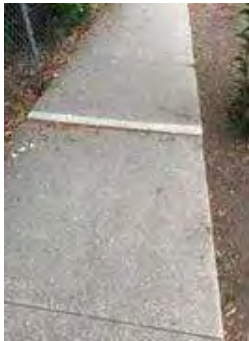
Hazard 22: 1335 Casitas Pass Rd
