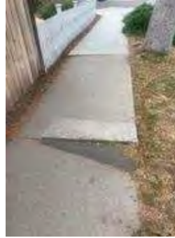
Hazard 11: 1492 Namouna St
