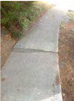
Hazard 2: 1547 Myra St
