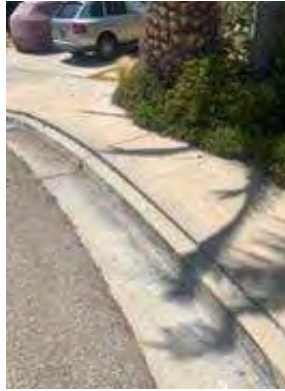
Hazard 1: 5004 Pacific Village Dr
