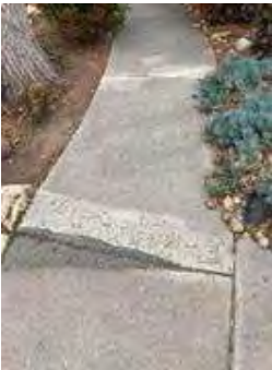
Hazard 8: 5410 Cameo Rd
