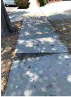
Hazard 10: 5390 Dariesa St
