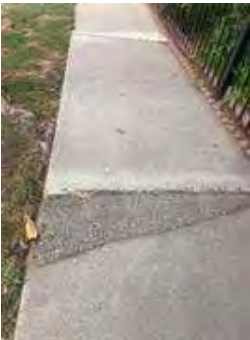
Hazard 3: 1476 Andrea St
